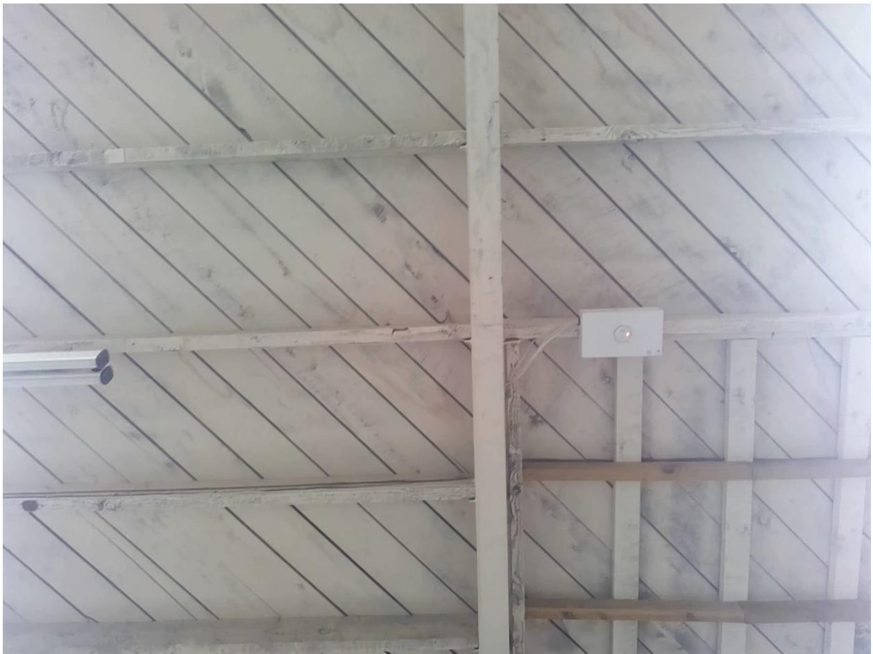
emergency lighting Taken at 1:42 PM on Friday 16/07/2021
