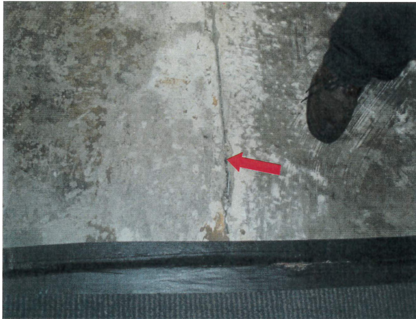
Photo 03: Crack at control joint in slab on grade
