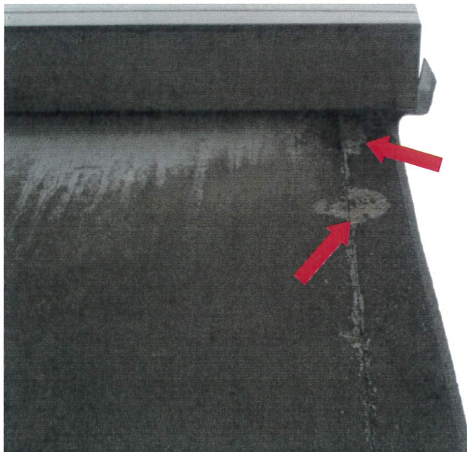
Photo 06: Spalls at exterior face of panel
