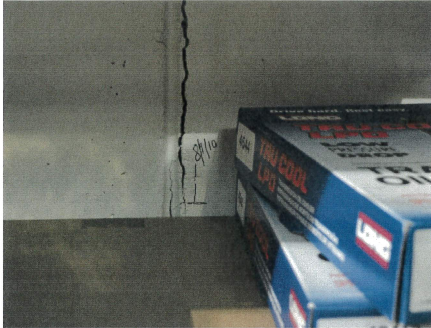
Photo 05: Separation between wall panels.
