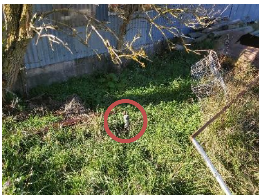
Figure 16: Buried petrol tank outlet
