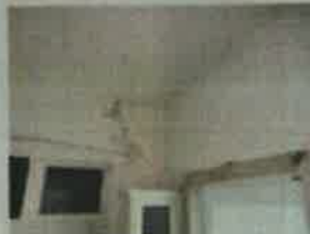
Figure 3: Superficial cracking in the interior of one of the Bays.
