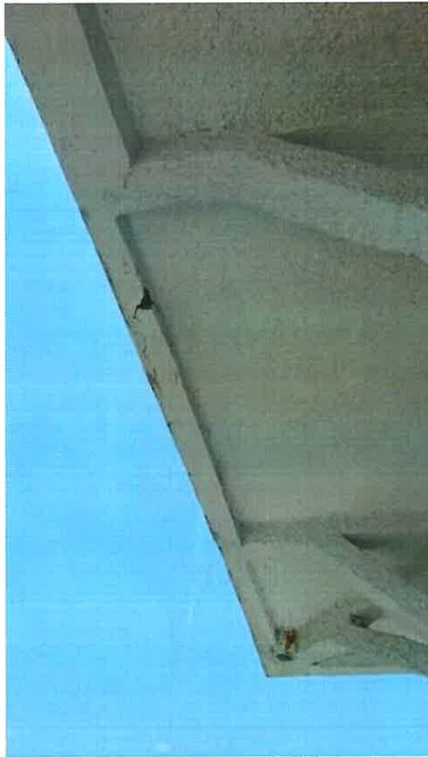
Concrete deck underneath flat B fractured
