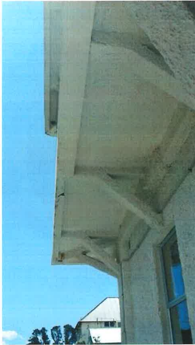
Concrete deck underneath flat B fractured
