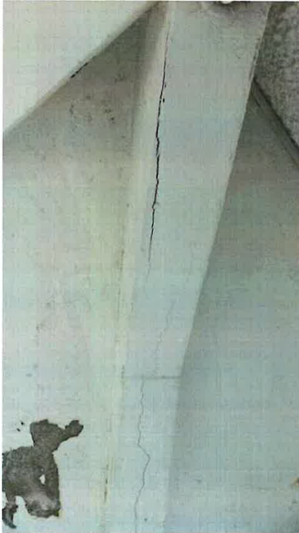
Concrete fracture to flat B entry, epoxy crack injection required.
