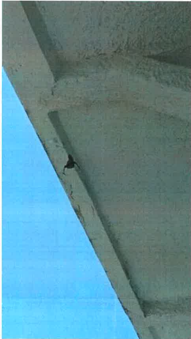
Concrete deck underneath flat B fractured
