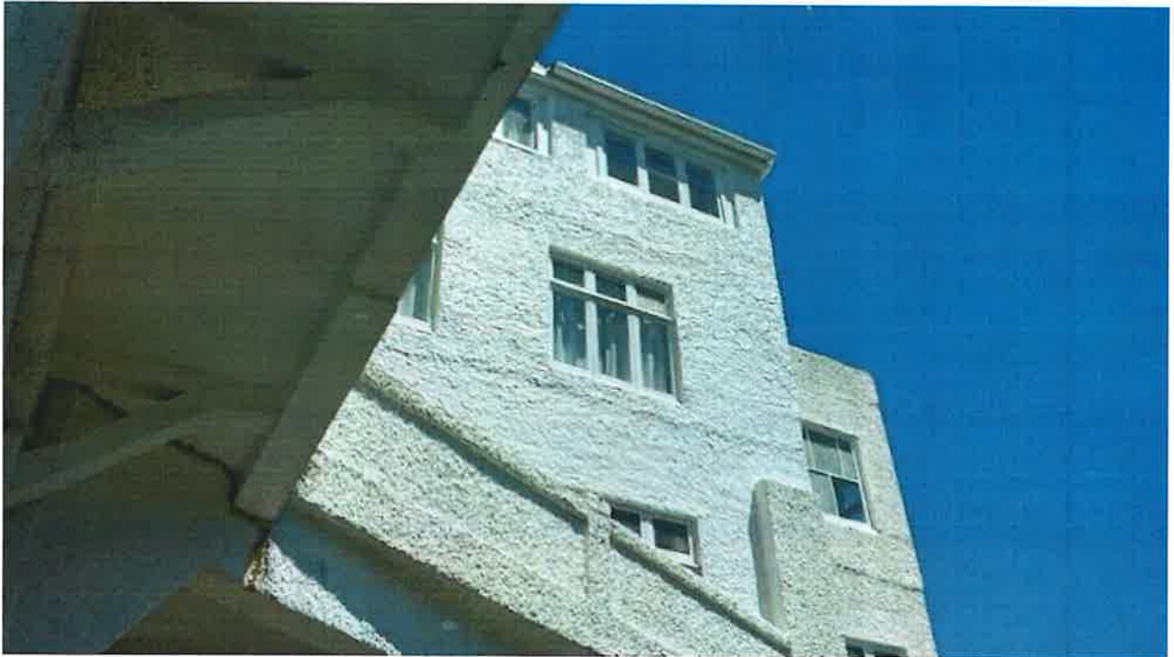
Multi complex building, damage assessed on flat B only
