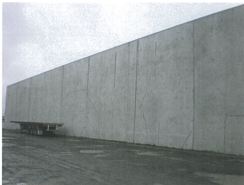
Figure 3: Cracking of boundary wall panels.
