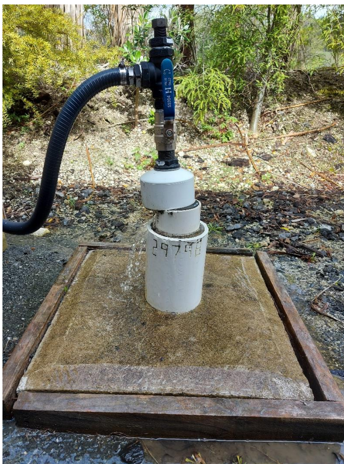
Figure C: Collar of Production Bore ID29798 showing Artesian Flow
