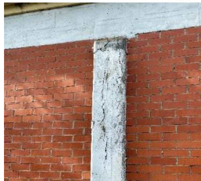
FIGURE 2 – BUILDING 4A CONCRETE COLUMN CRACKS
