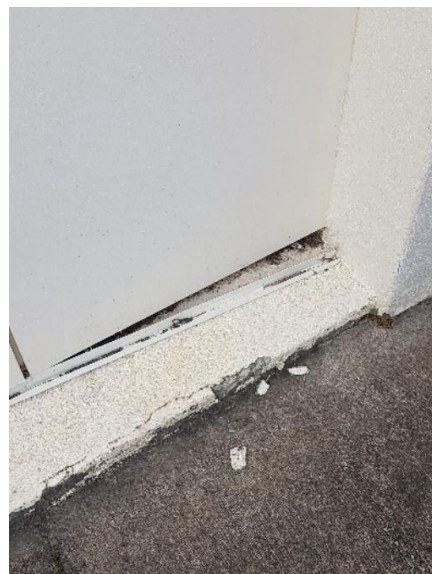
Figure 25: Damaged titan board on the Western façade.
