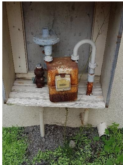
Figure 29: Rusty meter to be removed
