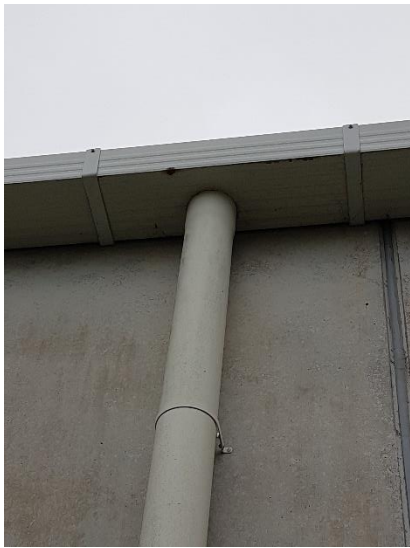
Figure 13: Edge of the beam box on the Southern Facade showing signs of corrosion.
