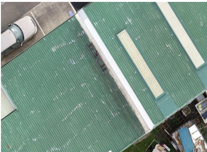
Figure 21: The Northern block roof is showing signs of deterioration, but the skylight panels appear to be in satisfactory condition.
