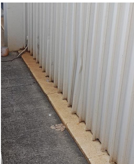
Figure 24: The Northern Block showing the profile iron cladding which is dented and signs of rusting at the bottom.
