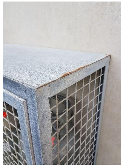
Figure 12: Gas cage located on the Southern facade showing signs of corrosion. (Tenant owned)
