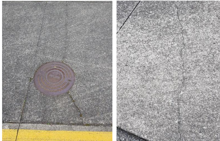
Figure 20: Concrete near Central Block showing some minor cracks.
