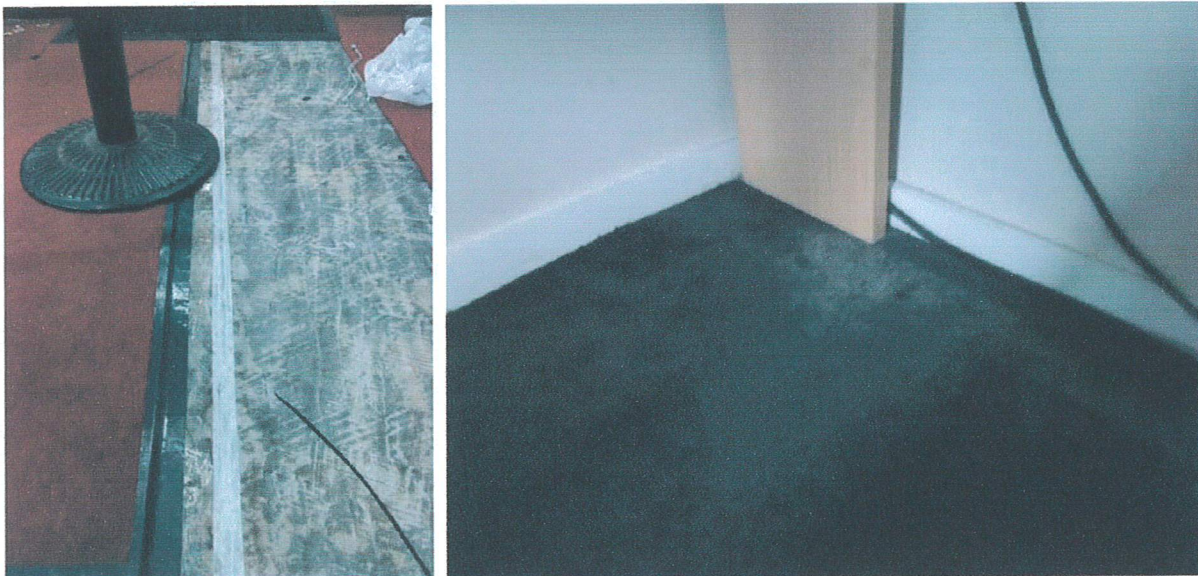
Unit 7 floor banding and liquefaction to existing carpet.
