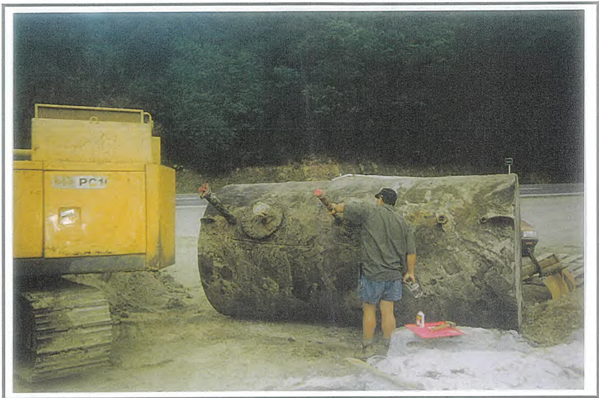
Photo 3: The second 9,000 litre diesel tank (TP2).
