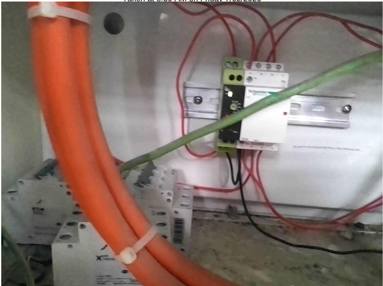
Emergency lighting test facility Taken at 8:40 AM on Friday 7/02/2020
