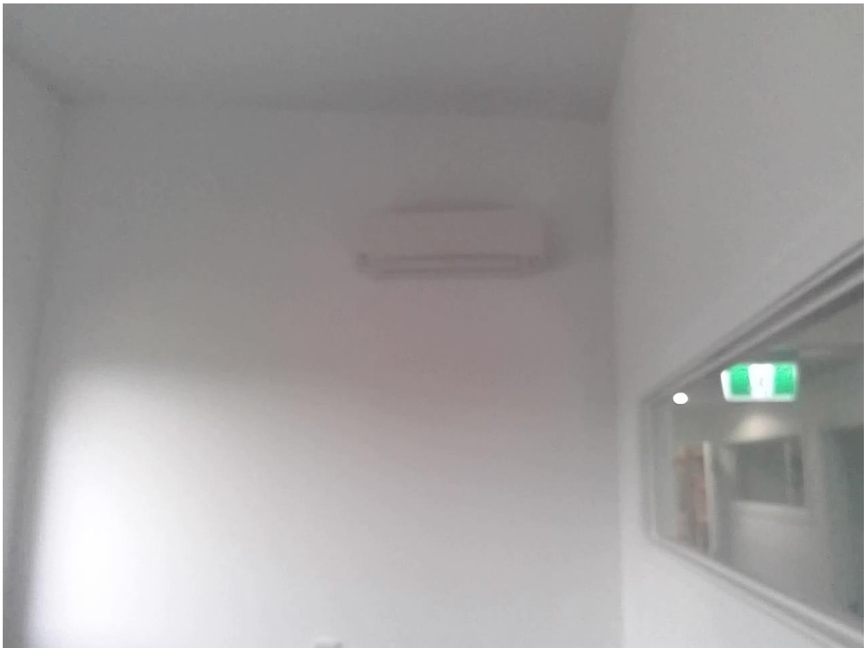
Heatpumps installed Taken at 8:54 AM on Friday 7/02/2020
