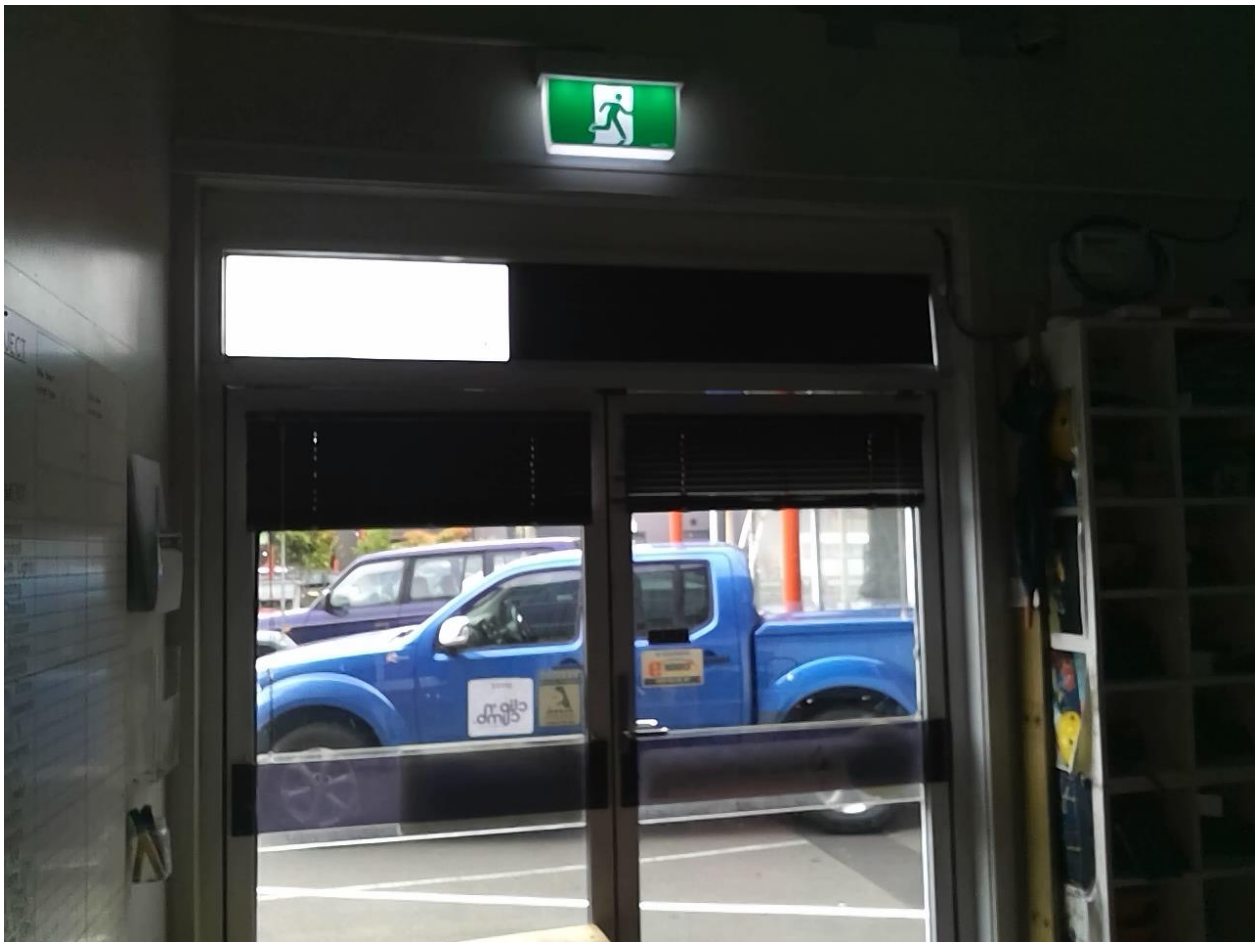
Illuminated exit sign + keyless lock installed @ existing office Taken at 8:42 AM on Friday 7/02/2020
