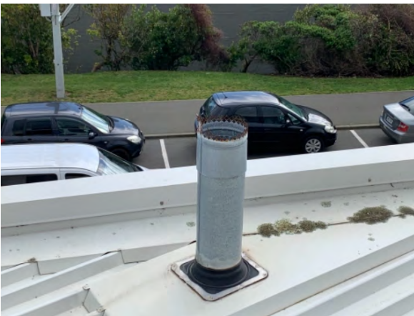
Missing roof cowl
