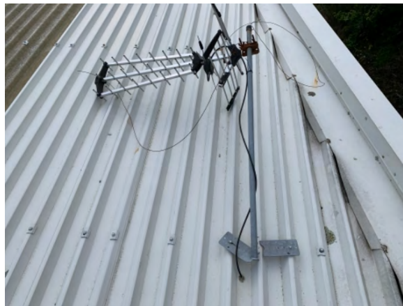
Broken aerial and mount Roof mounted aerial has broken off and is sitting on the roof. The mounting bracket has also broken.
