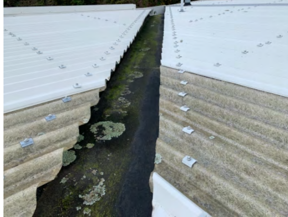
Moss and mould in gutter
