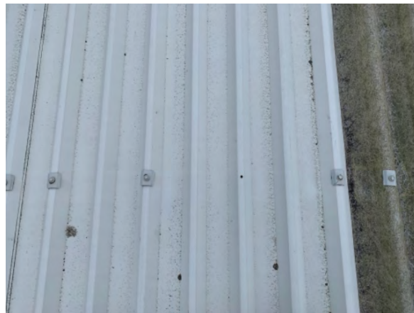
Missing screw and washer Example of an area where there are missing roof fixings and profile washers.
