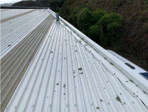
Moss on roof
