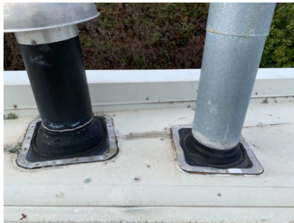
Penetrations with dektites faded sealant around dektite and missing clamp rings around the top.
