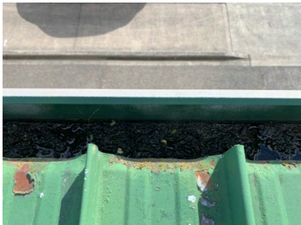
Debris in gutter
