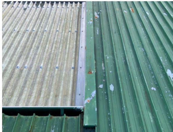
Surface rust spots on flashing
