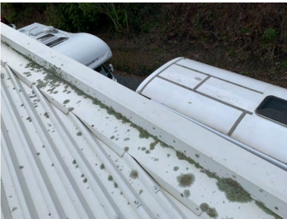
Moss build up on flashings
