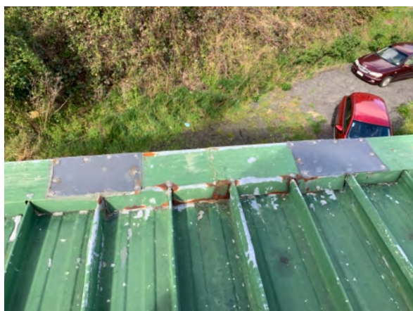
Corroded flashing with repairs
