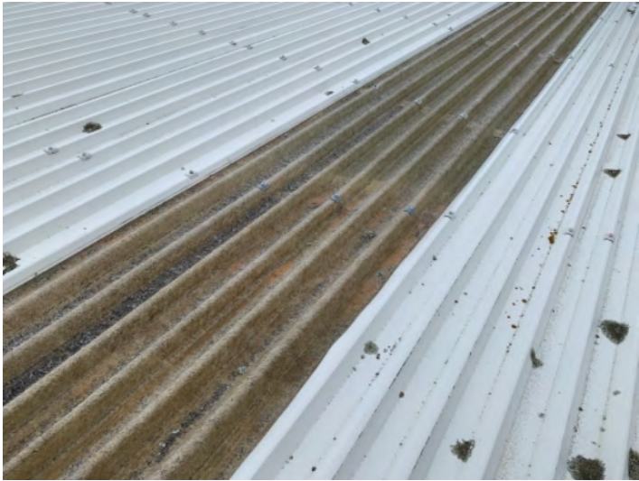
UV damaged and brittle skylights
