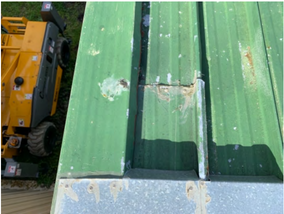
Faded sealant on short sheet
