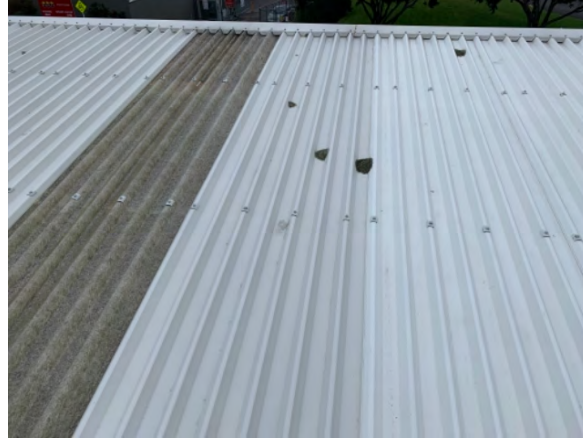
Two different sheet colors have been used on the roof. Possibly previous sheet replacement done.
