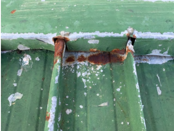
Rust on roof sheets
