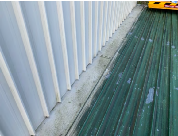
Moss and mould on flashing
