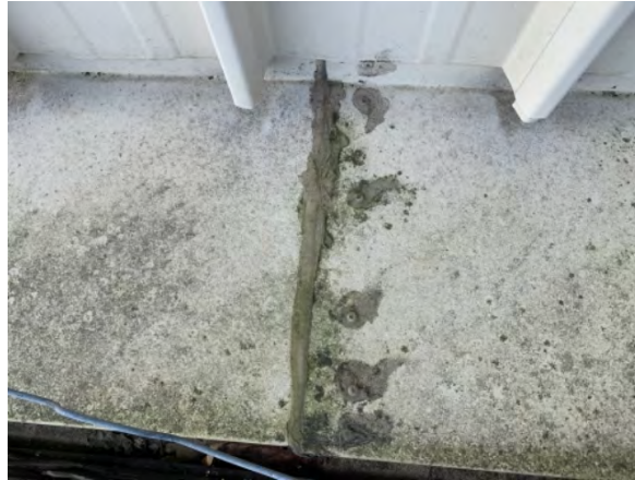
Faded sealant on flashings
