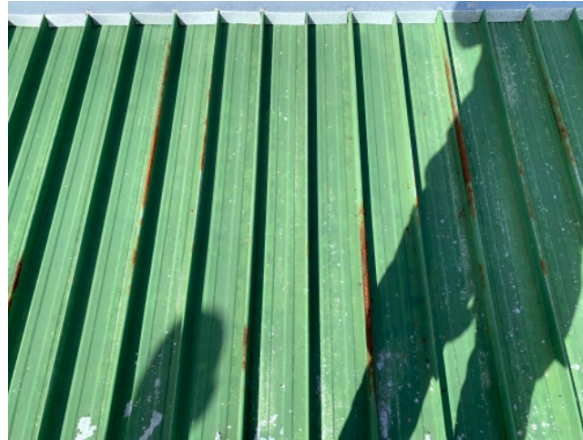
Corrosion on ribs
