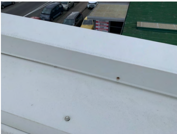
Missing fixing on cap flashing
