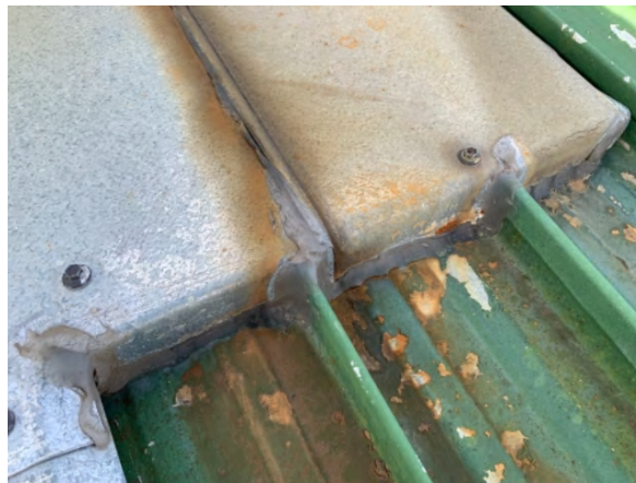
Previous sealant repairs
