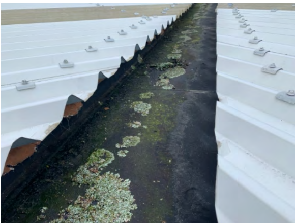
Moss and mold in gutter
