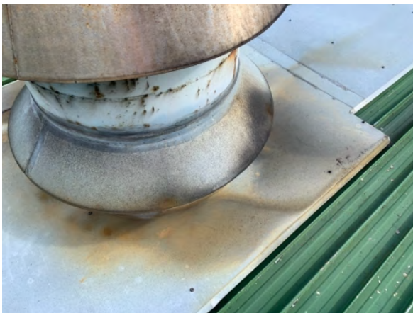
Stains on flashings
