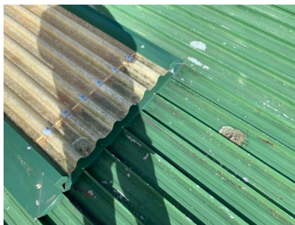
Moss on roof
