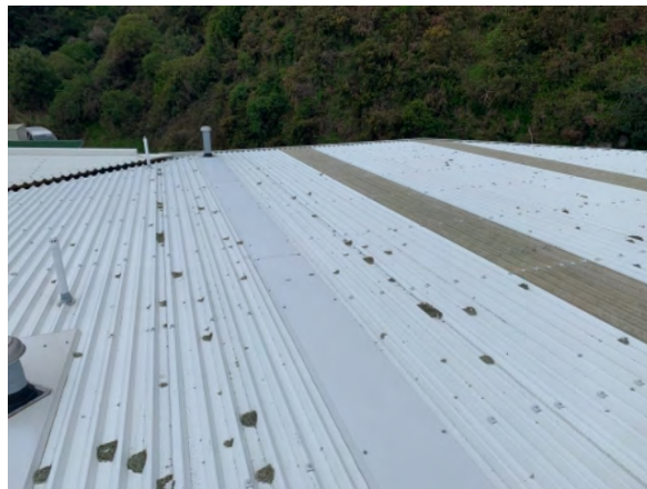
Moss on roof
