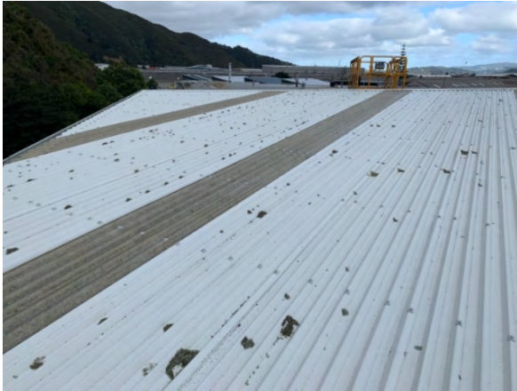
Moss on roof
