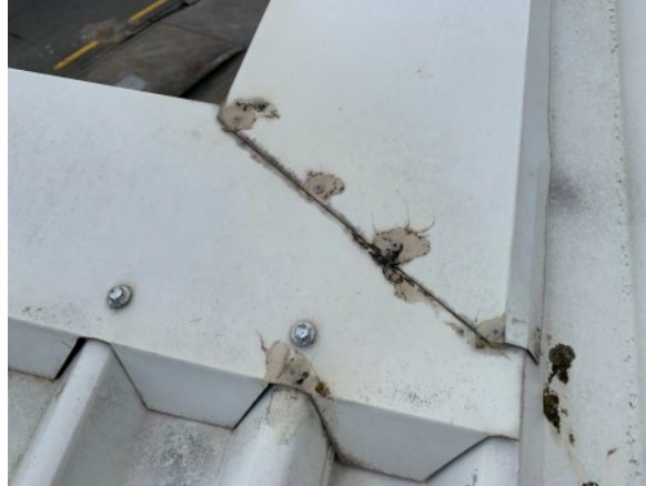
Faded sealant on flashings
