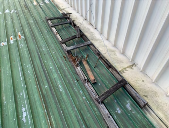
Old, rotten timber on roof
