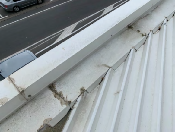
Faded sealant on flashings
