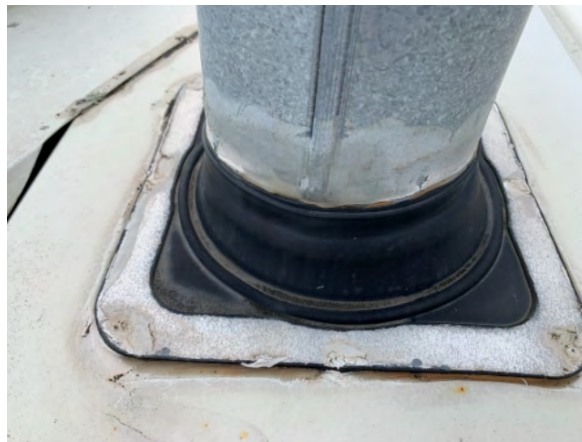
Faded sealant around Dektite
