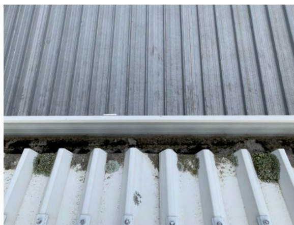
Moss and dirt build up at end of sheets There is a lot of moss and mold building up at the ends of the sheets going into the metal box gutter.
