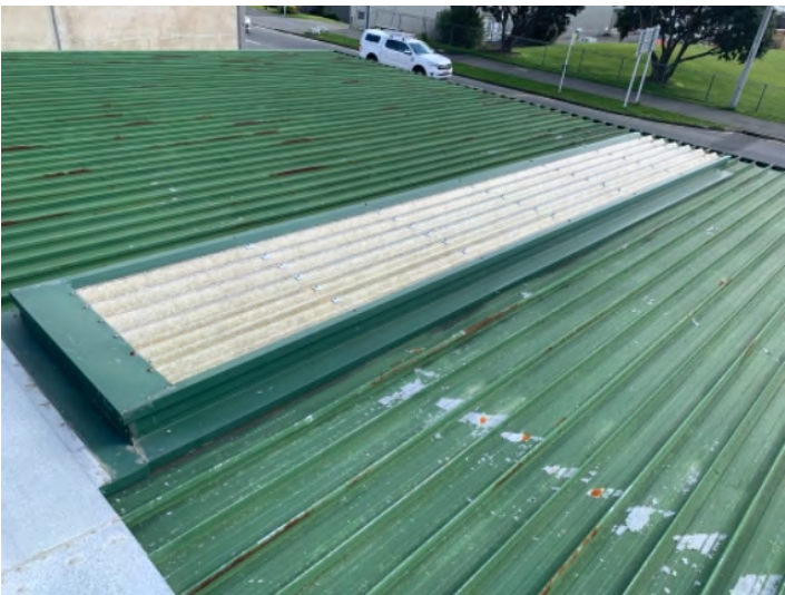
UV damaged and brittle skylights
