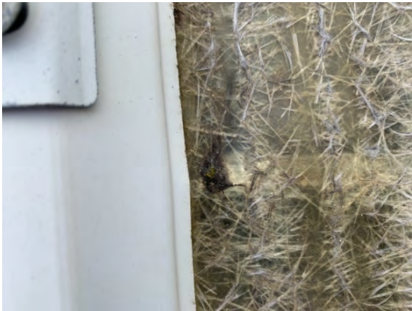
Hole in skylight
