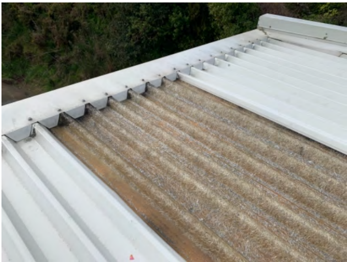
UV damaged and brittle skylights
