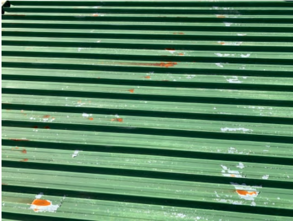
Corrosion spots on roof
