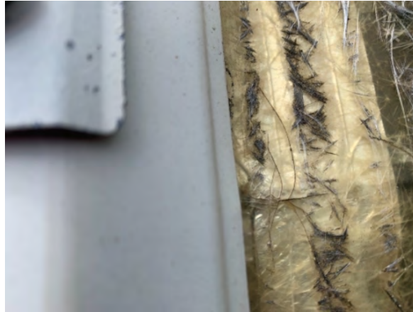
Fractures in skylight
