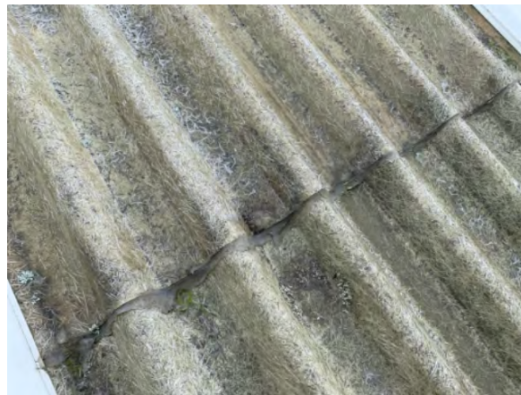
Sealant on skylight starting to fade The sealant in the junction where the two skylight sheets lap is starting to fade which can lead to water ingress by wind driven rain.
