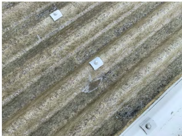
Previous skylight repair
