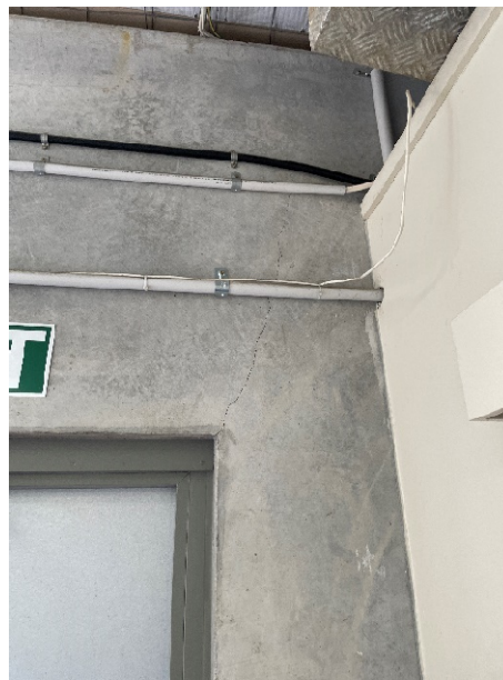
Photo 5: Cracking Observed at Re-Entrant Corner of Doors.
