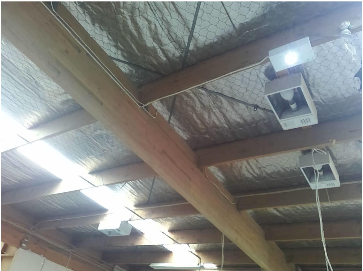
emergency lights tested Taken at 1:44 PM on Friday 16/07/2021
