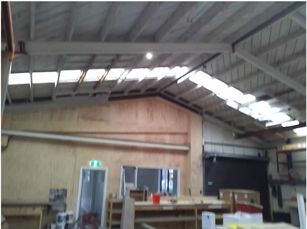
Emergency lighting + illuminated exit sign in warehouse Taken at 8:41 AM on Friday 7/02/2020
