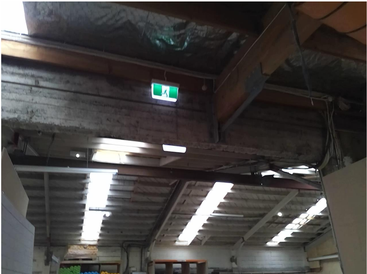
Illuminated exit sign in warehouse Taken at 8:52 AM on Friday 7/02/2020
