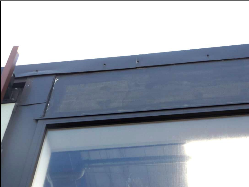
Western window showing poor application of paint
