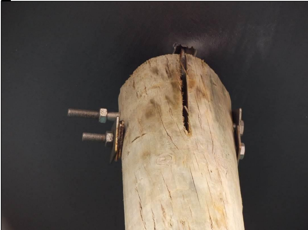
Showing the insecure pole fitting – noting the lack of thread length - Unit 55
