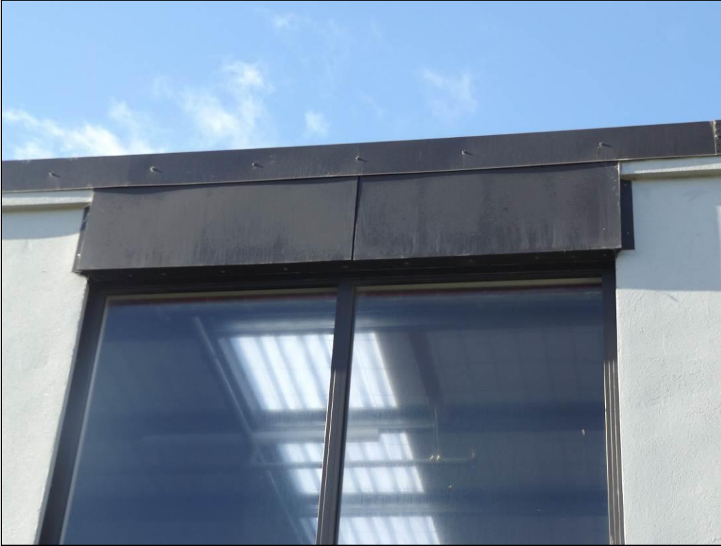
Showing an example of the poorly painted and uneven non aligned panels
