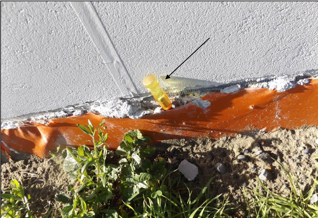
Western elevation showing the DPM which is turned up but not taken up under the rockcoat – note the chisel showing the access for water entry behind
