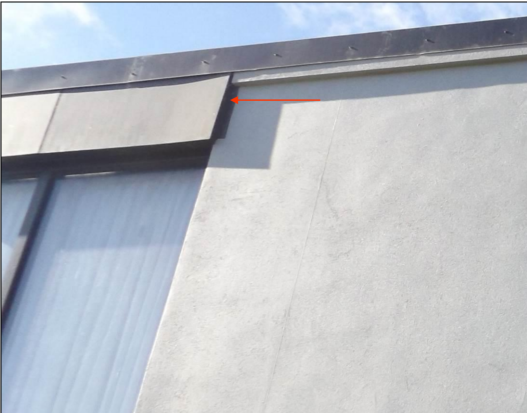
Showing an example of the proud brackets forcing the end of the panels out
