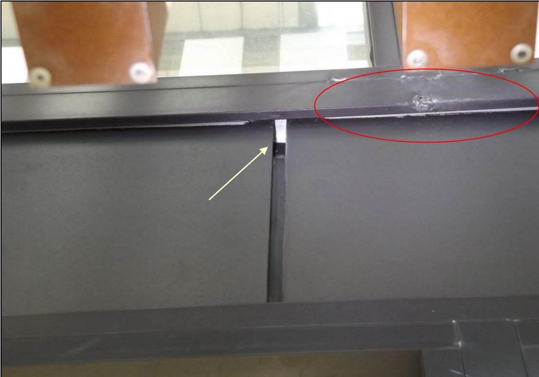
Showing how sealant installed between joinery panels doesn't extend to close the gap and salt deposits clinging to the joinery frame
