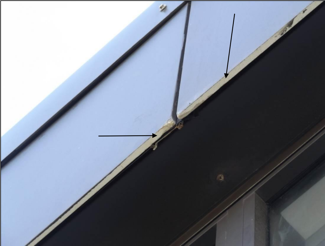
Showing the bottom and likely the sides of the panels are unpainted
