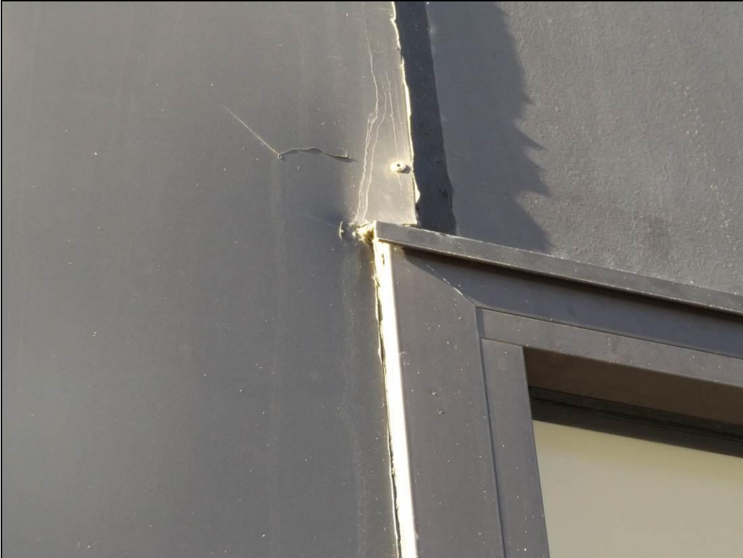
Western window – Bent flashing with reliance on sealant to provide protection to a bent joint – note the short head flashing detail and thin bead of sealant
