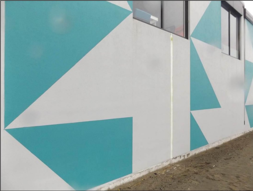
The remaining cracks extend from window sills
