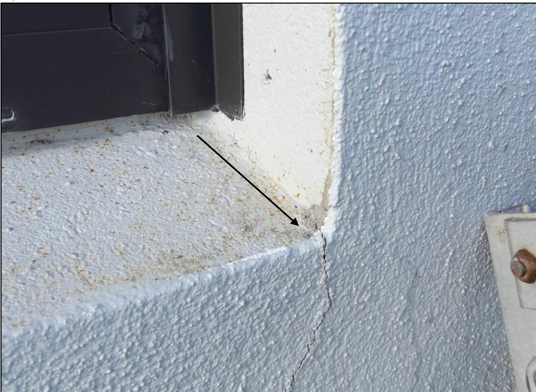
Showing the difference in materials and the ridge created by the repair and unsealed concrete allowing water to get down behind into the wall and behind the Rockcoat plaster delaminating it.
