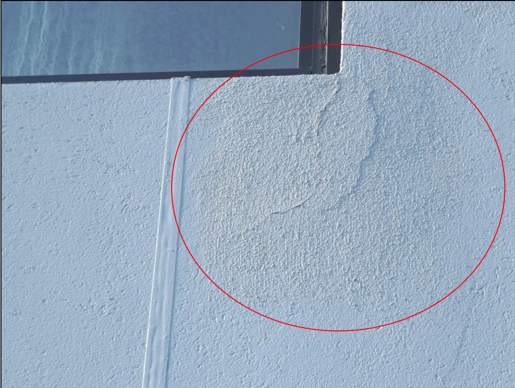
Showing an area that has re-cracked after repair (repair noted by the shadow)
