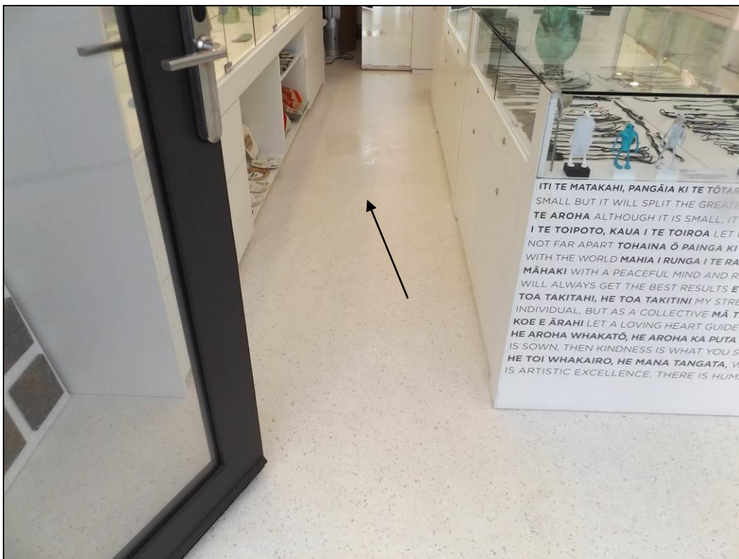
Unit 55 – showing the water on the floor from the leak
