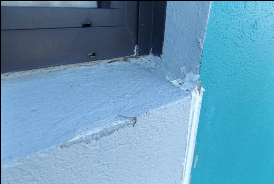
Showing damaged Rockcoat and a partially repaired crack on the outter edge of the sill
