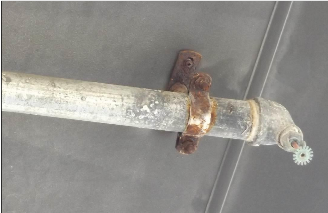
Showing a corroded sprinkler bracket and the white and red corrosion forming on the galvanised pipe - Units 23, 24
