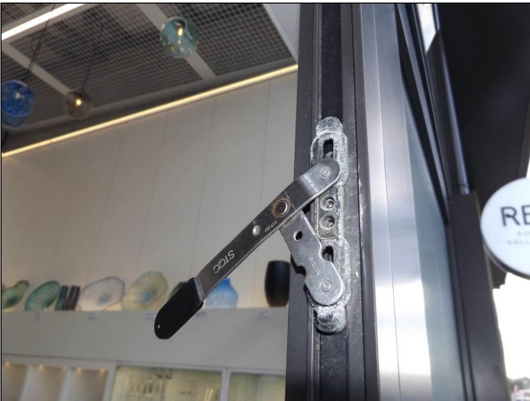
A double door fastening lever – In my opinion very flimsy engineered construction and noting the obvious formation of corrosion on the non-stainless part of the clasp
