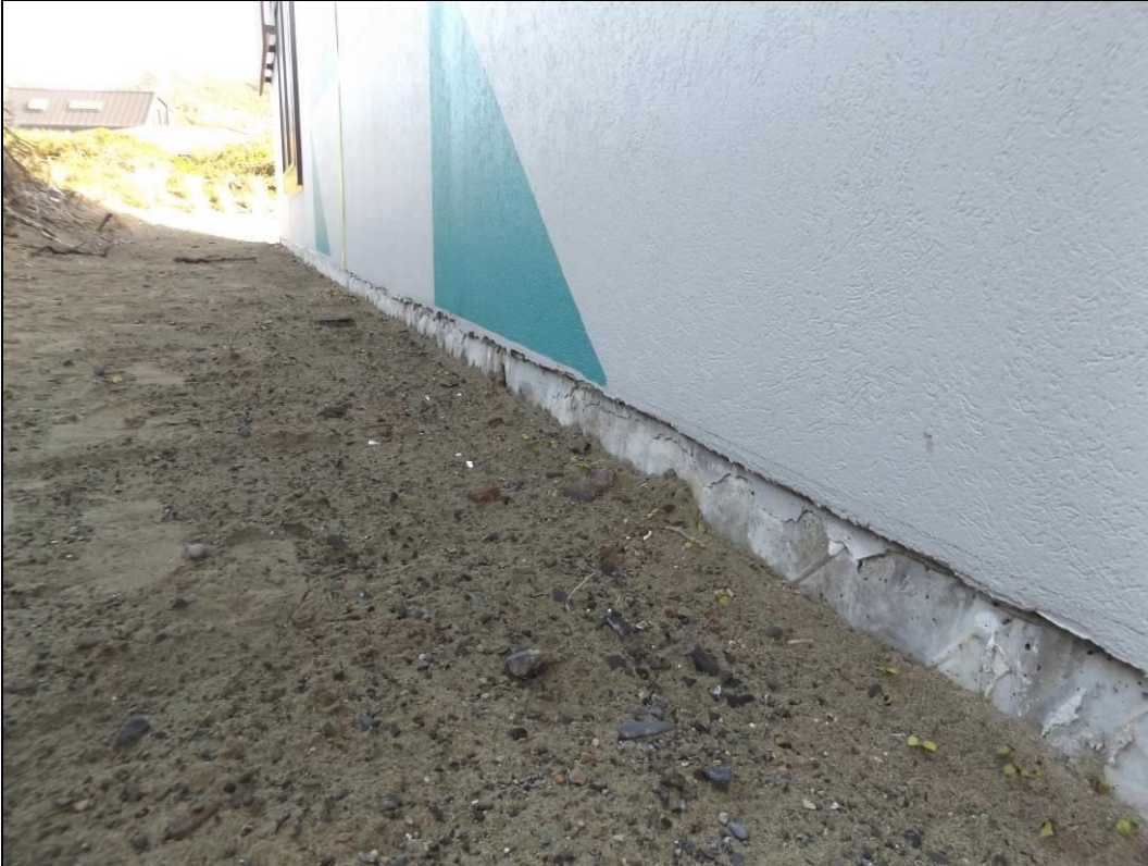
Southern elevation - Showing the unprotected foundation and junction with the Rockcoat – note the sand and sand dune located to left of photo
