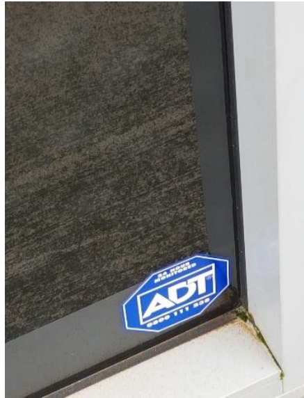
Figure 11: Window from the Southern Block with some build up in the corner.
