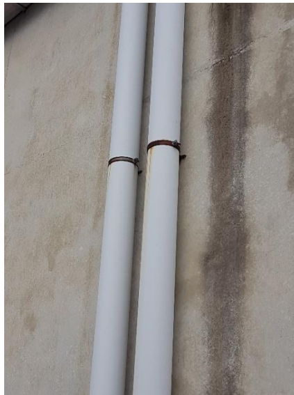
Figure 19: Rusty pipe brackets located on the North facade.
