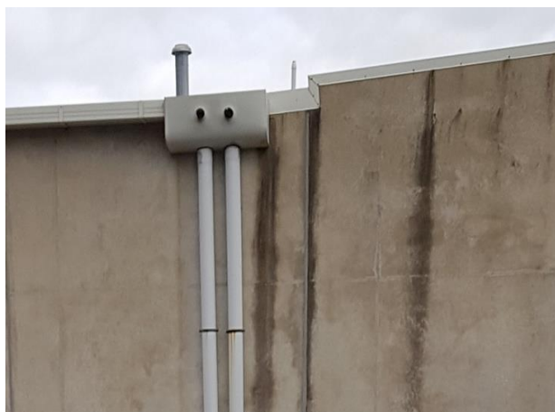
Figure 16: The northern facade of the Central block with visible water stains on the cladding.
