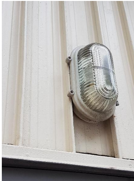
Figure 30: Bulkhead light with a crack. (Tenant owned).
