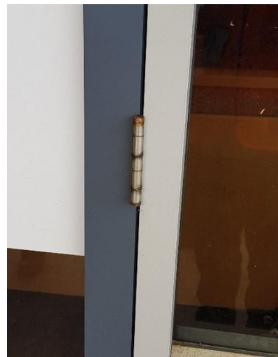
Figure 27: The front door located on the Western facade with signs of corrosion to the hinges.
