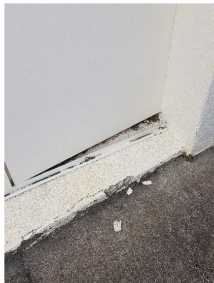
Figure 25: Damaged titan board on the Western façade.
