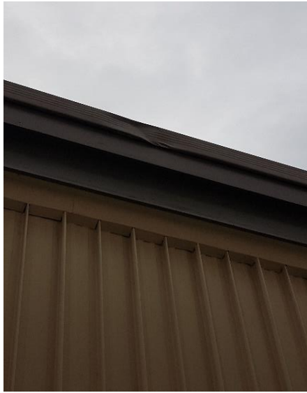
Figure 23: Box guttering with a dent in the Northern block.
