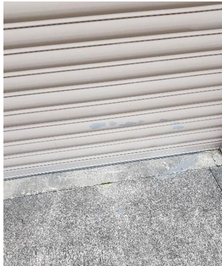
Figure 9: Minor paint chipping on the garage on the North Facade.
